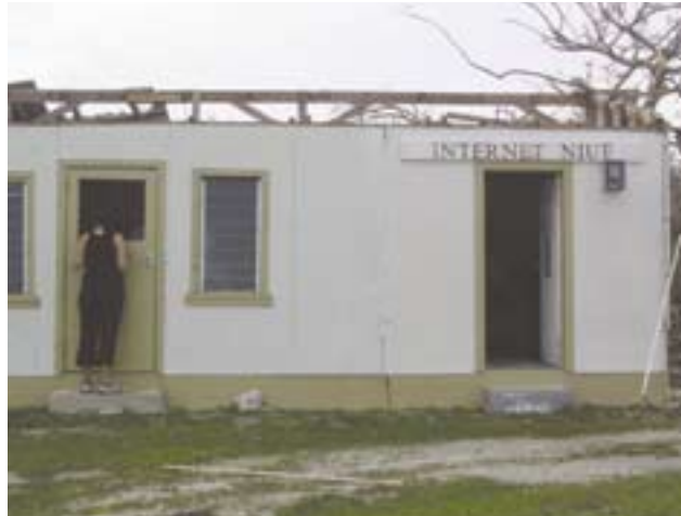
Inspecting the damage to ISU-N's Internet Cafe.
