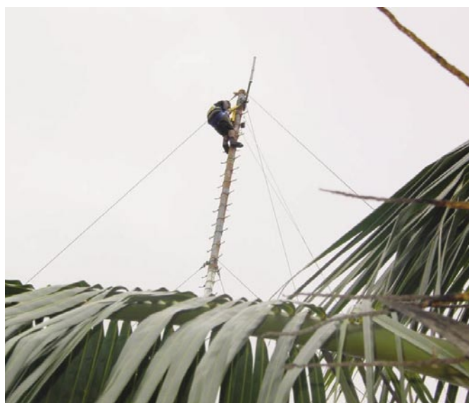
Emani Lui climbs to the top of the 120 foot high tower overlooking the village of Hakupu to install the WiFi Access Point.
